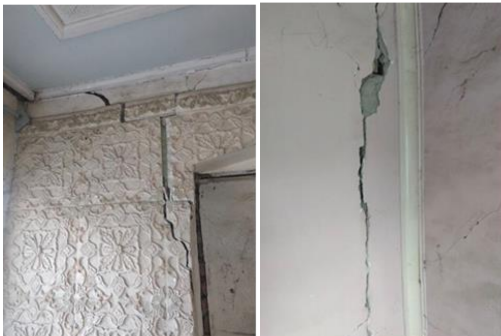
Figure 7. Old and new cracks on the wall of a house in Goyam village
