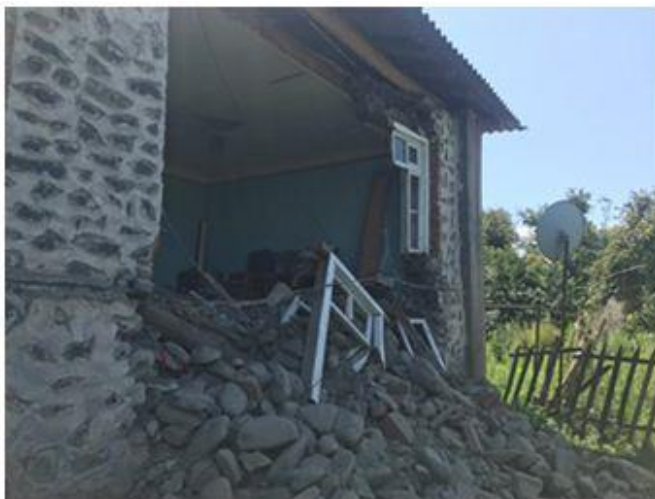
Figure 5. The collapse of the river stone wall of a house in the village of Makov
