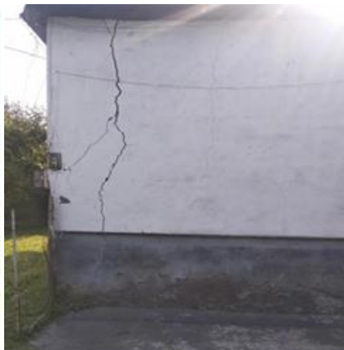
Figure 6. Old and new cracks on the wall of a house in Goyam village
