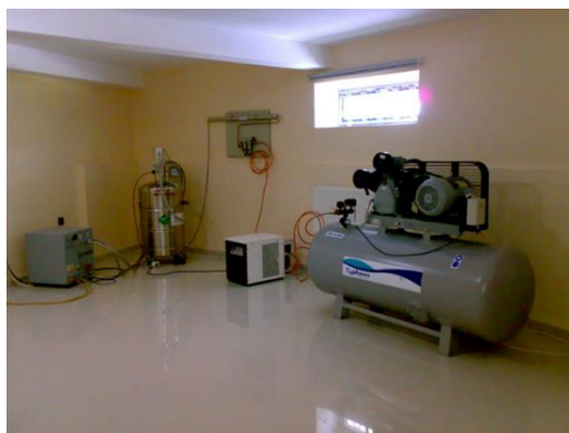
Liquid Nitrogen Plant LNP-20.
